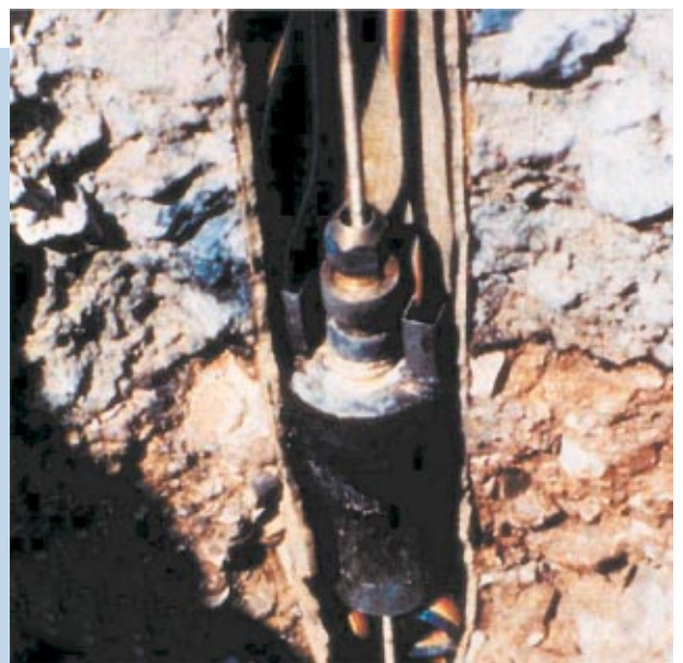
MULTI-DEPTH DEFLECTOMETER (MDD)
